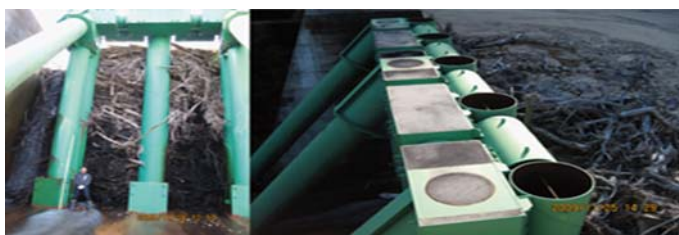
Figure 2. Sediment and driftwood trapped by the open check dam (beam type) in the Hachimandani River.
