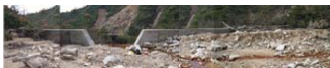
Figure 1. Sediment deposition caused by the closed check dam in the Tsurugi River.
